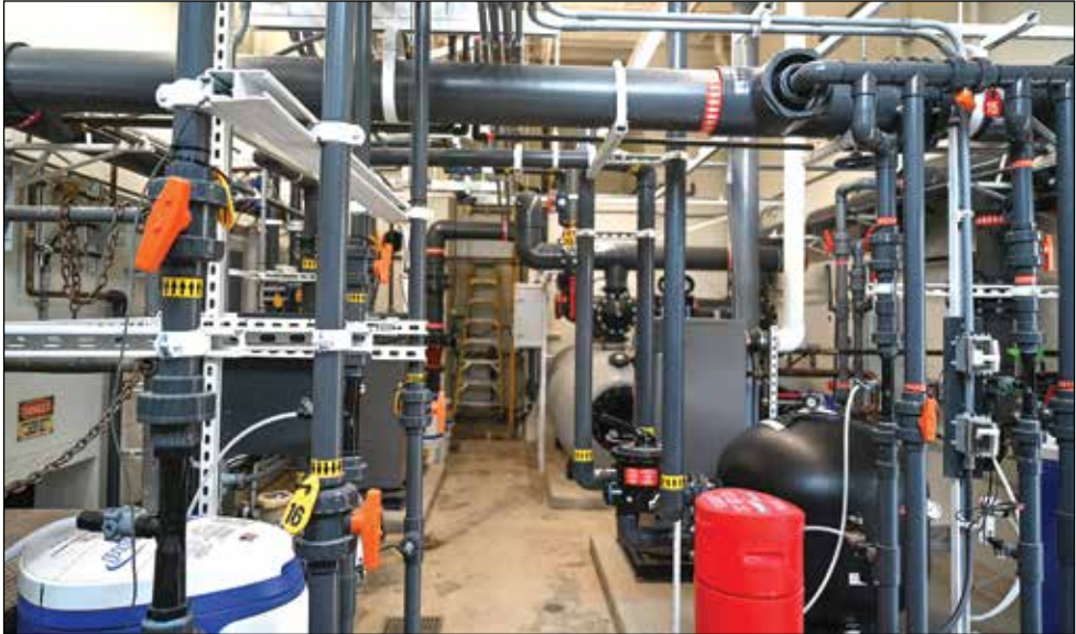
Everything is now shiny and new in The Plunge’s equipment room.
