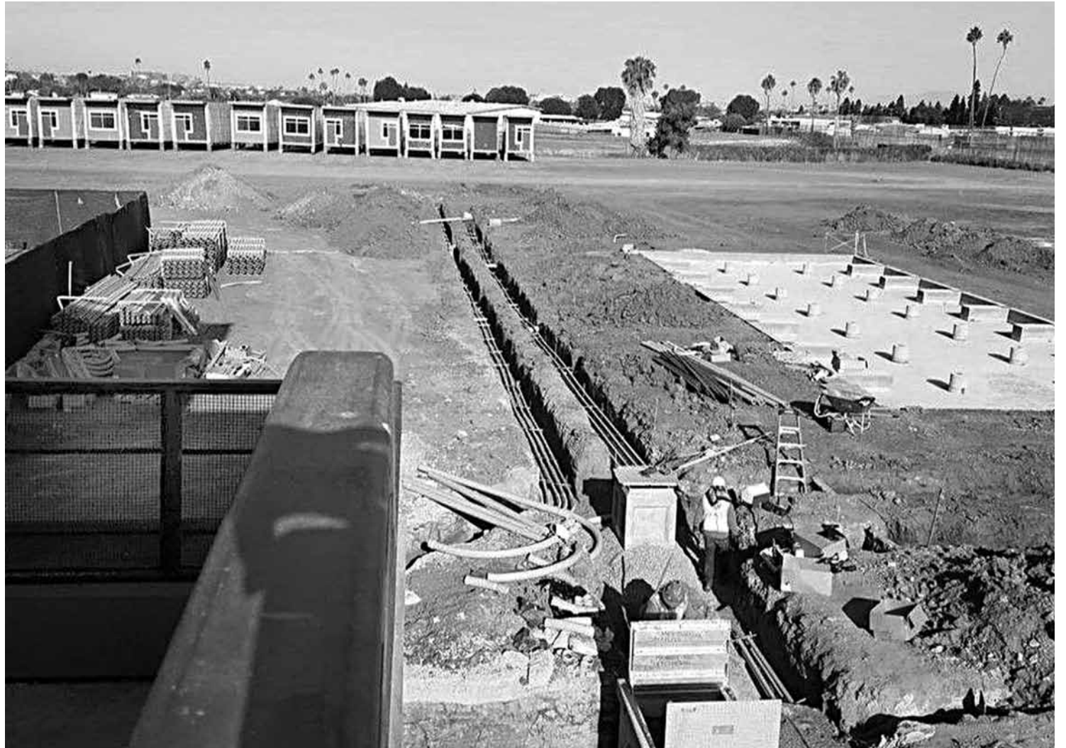
Last week, eight of the 16 new modular classrooms arrived at the Woodworth-Monroe TK-8 campus. Let the improvements begin! Photo: Inglewood Unified School District
