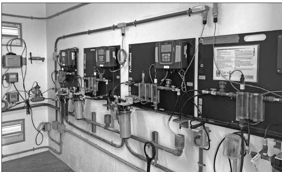
Online Water Quality Analyzers. Images Provided by Golden State Water Company.
